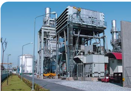
LM2500 industrial gas turbines provide the power supply for this natural gas compressor station.
