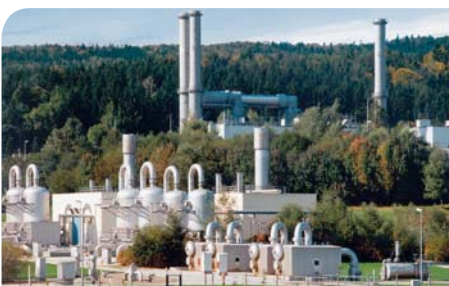
Industrial gas turbines are also used to power natural gas compressor stations.
